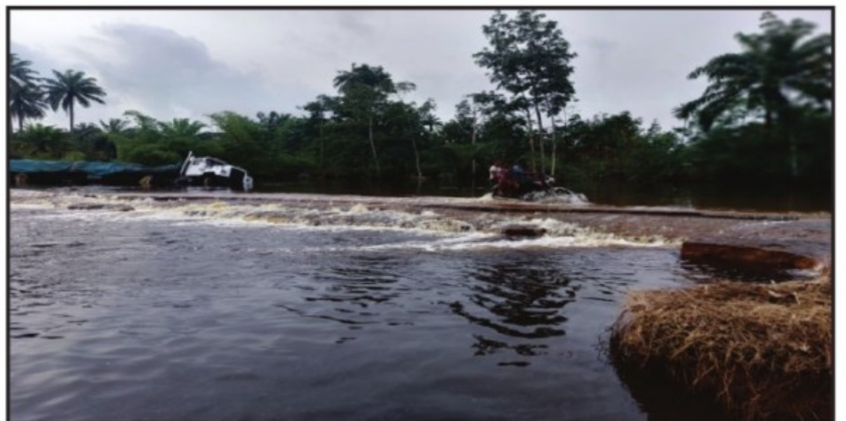
Portion of the East-West road at Ahoada swept away by the raging flood. Credit: Ibiba DonPedro
