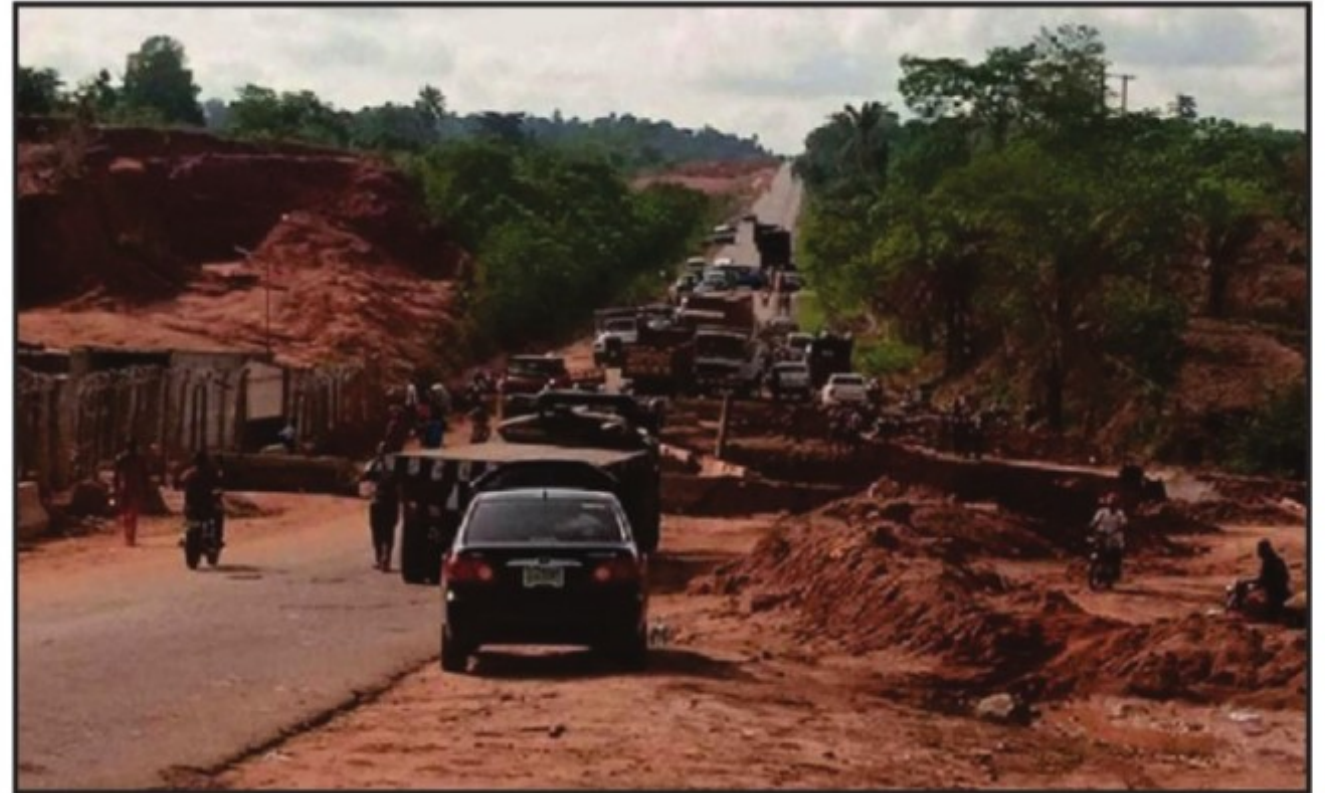
Collapsed portion of the Ughelli-Asaba Road
